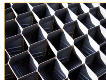
Honeycomb filters in Bio-tower
