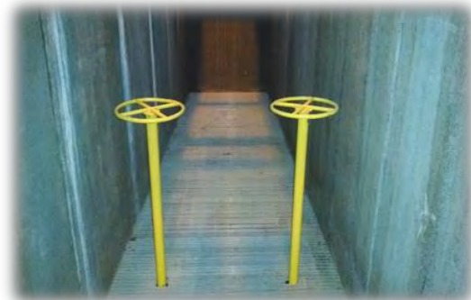
Above Ground Valves
