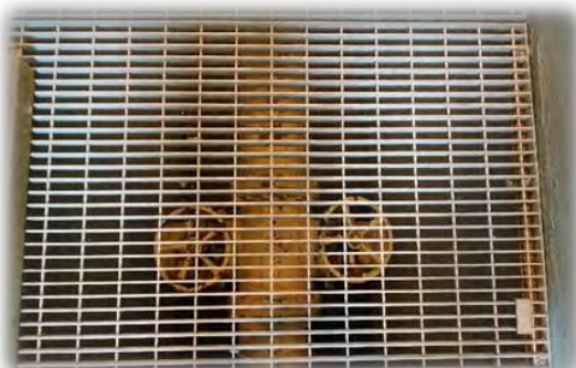
Below Ground Valves
